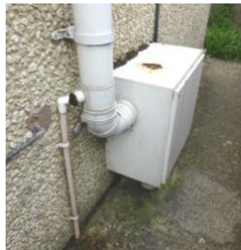
Q16 – Example of Radon Pump (to 1 No in Badgers Way, and 3 No in Woodpecker Way)
