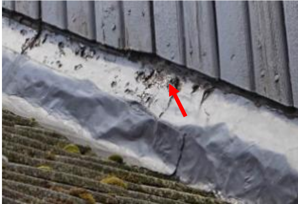
T19 – 3 Bushey Beeches, The Camp. Flashing at junction of Outbuilding & main house. Original flashing covered by “flashband” type repair, starting to disintegrate (arrowed)
