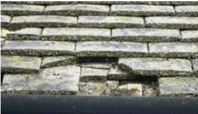
T29 – 8 The Knoll, Uley. Outbuilding front, slipped & missing roof tiles
