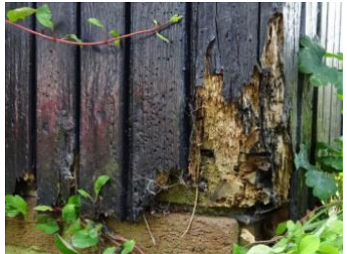
T32 – 3 Mount Pleasant, Wotton-Under-Edge. Front corner, rot & woodworm to outer boards & keel plate.
