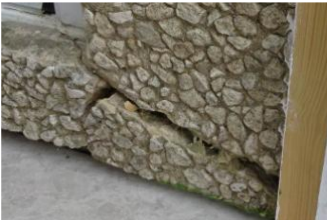
Q9 – 6 Badgers Way, Forest Green, broken panel section to right of front door (within porch)
