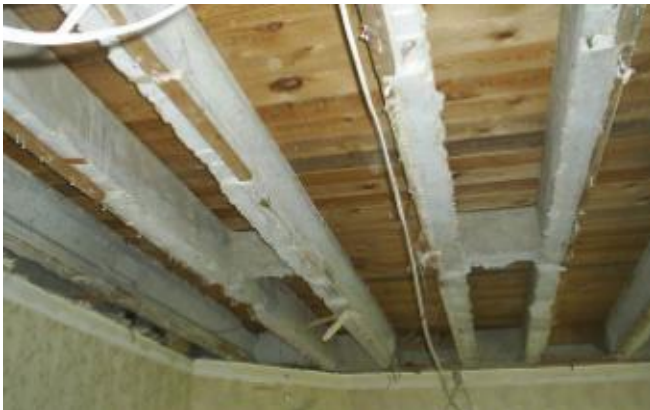
S49 – View of typical PRC “ladder” beams from below (not SDC stock photo)
