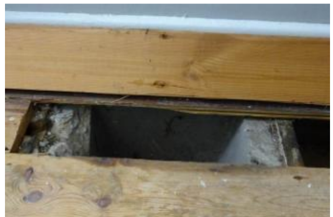
S48 – 6 Upper Park Road, Nailsworth. First floor construction, PRC ladder beams (see S49 for general view, taken in another house not in SDC stock)
