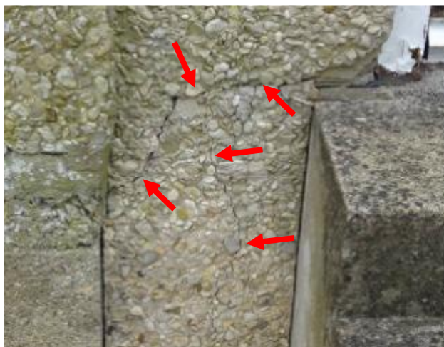
S41 – 6 Upper Park Road, Nailsworth. Cracking at dpc to side of door
