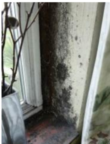
S29 – 39 Mankley Road, Leonard Stanley. Mould in window reveal at sill
