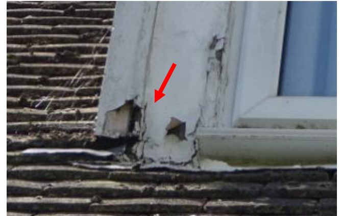
T36 – 3 Mount Pleasant, Wotton-Under-Edge. Rear dormer window poor paint finishes to framing & architrave
