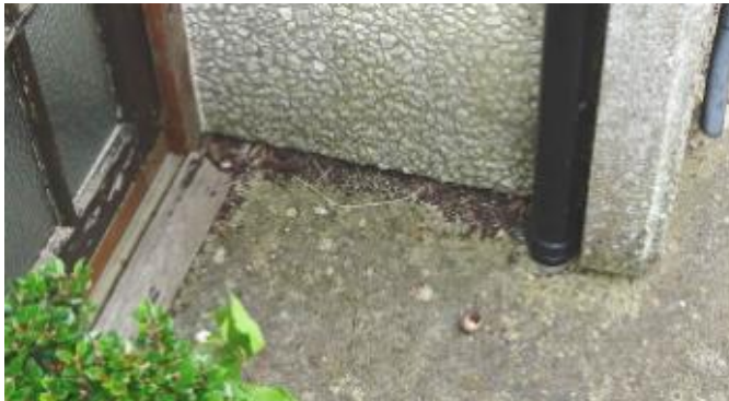
Q13 – Example of porch door away from rainwater downpipe & corner
