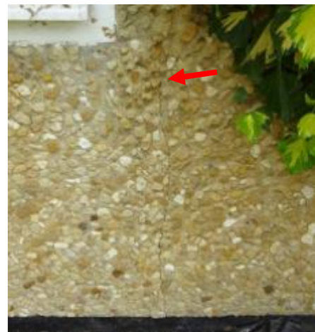
S71 – High Field, crack under front window
