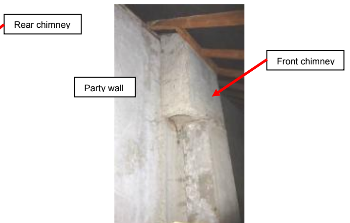
S54 – 6 Upper Park Road, Nailsworth. General view in loft towards party wall showing front chimney.
