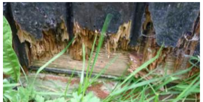
T10 – 32 Barrs Lane, North Nibley. Outbuilding side, rotten timber outer boards & keel plate
