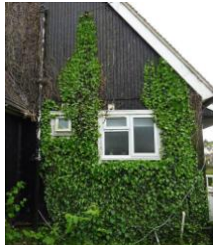
T8 – 32 Barrs Lane, North Nibley. Side, extensive ivy growth
