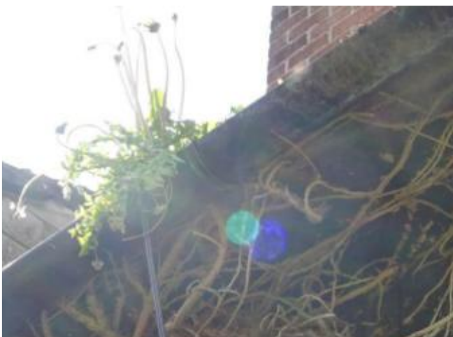
T41 – 7 Mount Pleasant, Wotton-Under-Edge. Rear, gutter vegetation & dead/dormant ivy growth
