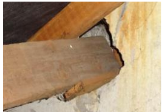
S52 – 3 Upper Park Road, Nailsworth. Roof purlin at party wall. Hole through to other side of wall, risk of fire spread.
