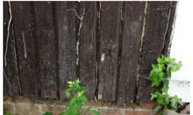
T28 – 6 The Knoll, Uley. Rear, example of rot & split outer boards near party wall
