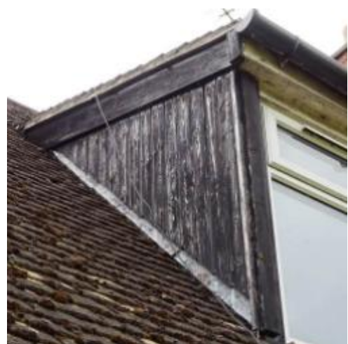
T12 – 32 Barrs Lane, North Nibley. Rear, poor timber to dormer side and architrave
