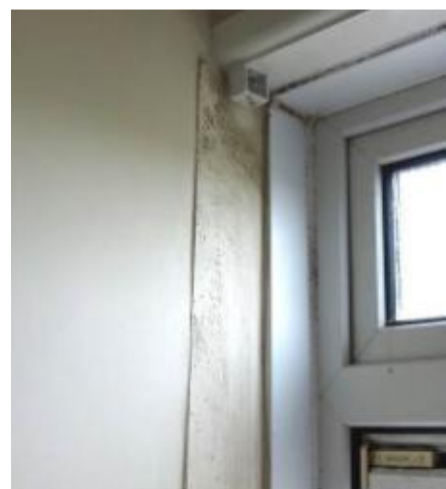
Q12 – 19 Nortonwood, Forest Green, mould in bathroom in window reveal
