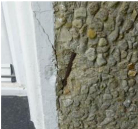
S27 – 56 Lawnside, Forest Green, front spalling to right of front door. Corroded steel & crack
