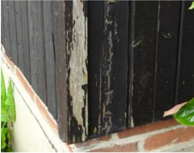
T25 – 6 The Knoll, Uley. Rear, rot to bay window corner architrave
