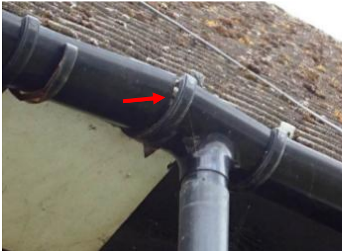
T7 – 32 Barrs Lane, North Nibley. Front gutter disconnected at downpipe bracket (arrowed)
