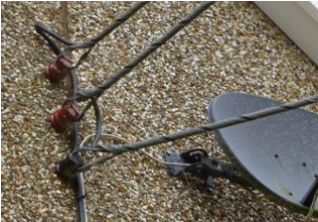
S37 – 38 Glebe Road, Minchinhampton. Overhead electric cables to gable
