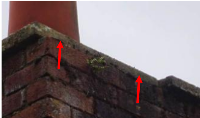
T13 – 32 Barrs Lane, North Nibley. Rear party wall chimney capping broken away (arrowed)
