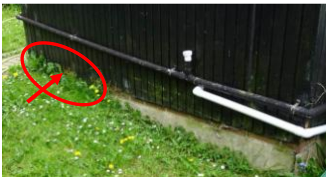
T9 – 32 Barrs Lane, North Nibley. Outbuilding side, ground level too high (circled). Rot to outer boards at dpc level (T10 circled)
