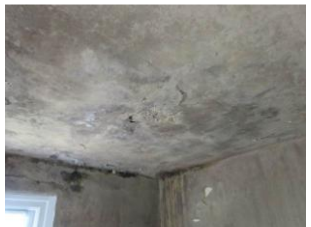
S66 – 31 Victory Road, Whiteshill. Side extension general view of concrete ceiling (note: S67 is just off picture to right)
