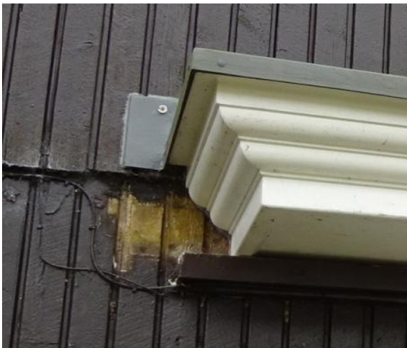
T21 – 6 The Knoll, Uley. Front, replacement canopy leaves untreated timber outer boards
