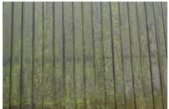
T18 – 3 Bushey Beeches, The Camp. Side elevation, algae growth on outer boards
