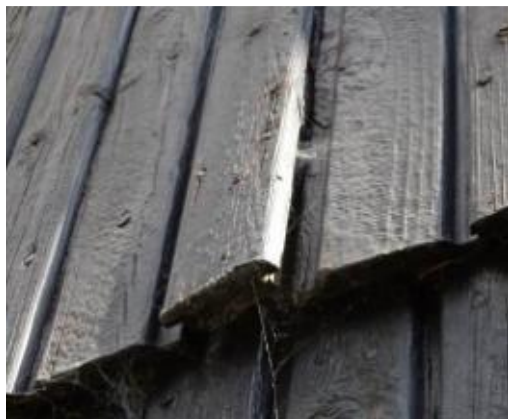
T17 – 3 Bushey Beeches, The Camp. First floor outer boards, board “sprung” due to failed fixing
