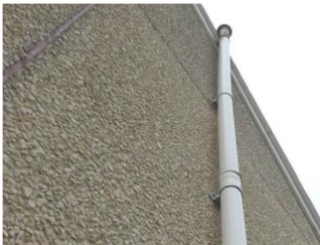
Q17 – Example of Radon ducting from pump
