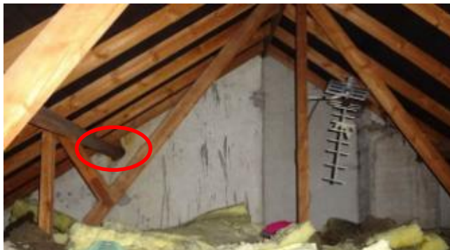
S51 – 3 Upper Park Road, Nailsworth. General View in Loft towards the party wall (S52 circled)
