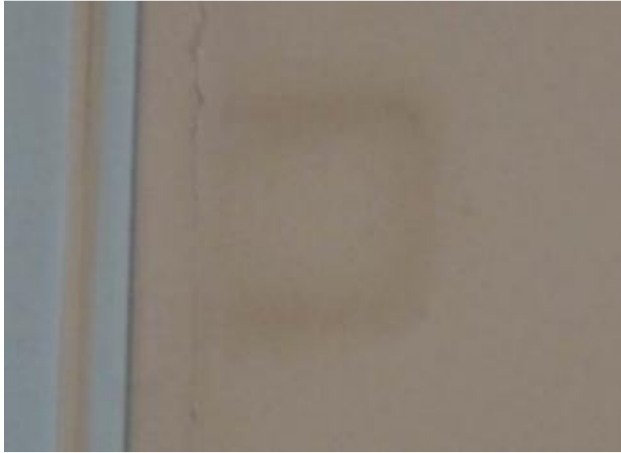
S25 – 45 Lawnside, Forest Green, bedroom gable wall, left hand staining detail
