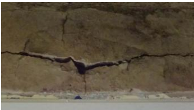
S65 – 31 Victory Road, Whiteshill. Side extension cracking above window viewed internally, detail
