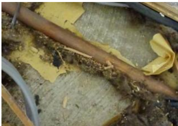
S47 – 3 Upper Park Road, Nailsworth. First floor, suspended cast in-situ concrete slab under floorboards and battens.
