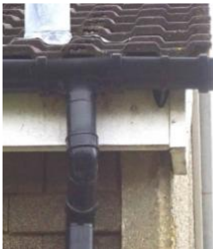
Q15 – Example of roof verge close to external wall (need to extend roof for EWI)
